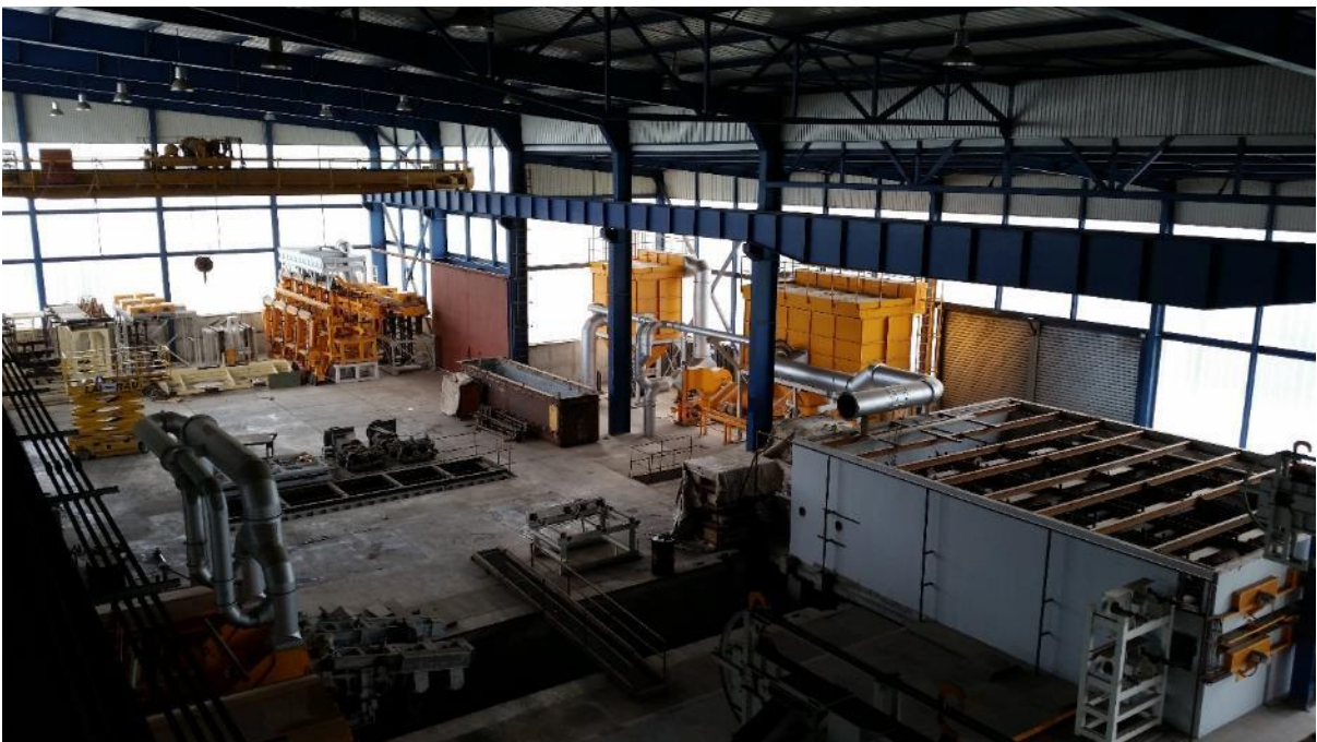
Zinc – coating Section
