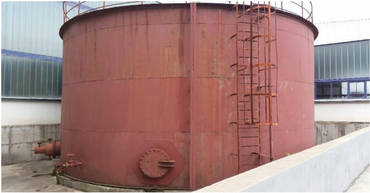
Tank for hard fuel (mazut)
