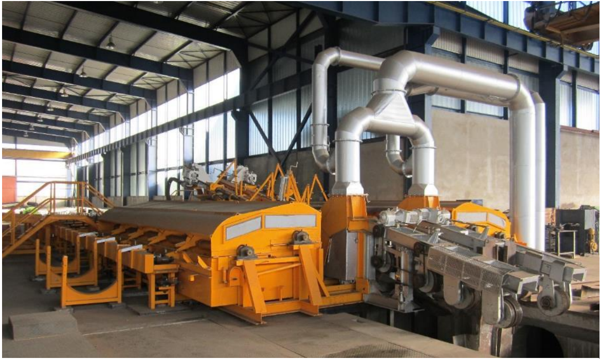
Magnetic rollers and pipe extraction machine
