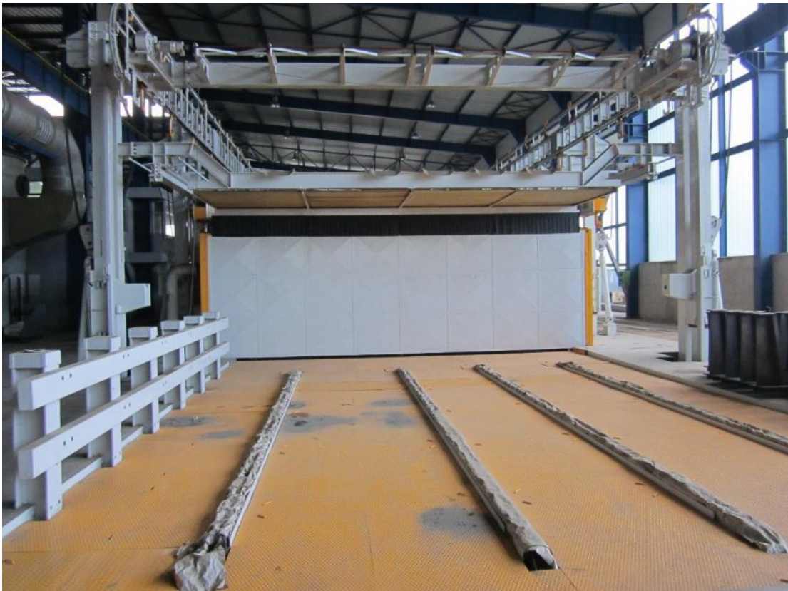
Chain transporters - Entry section
