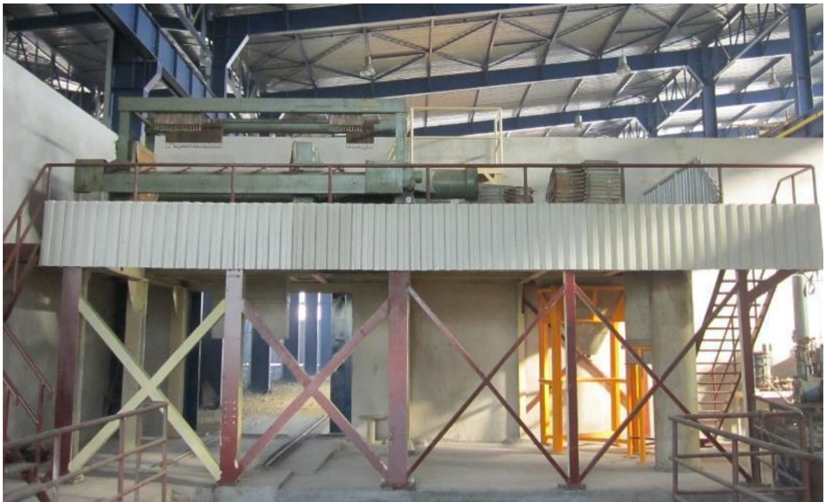
Water neutralization plant
