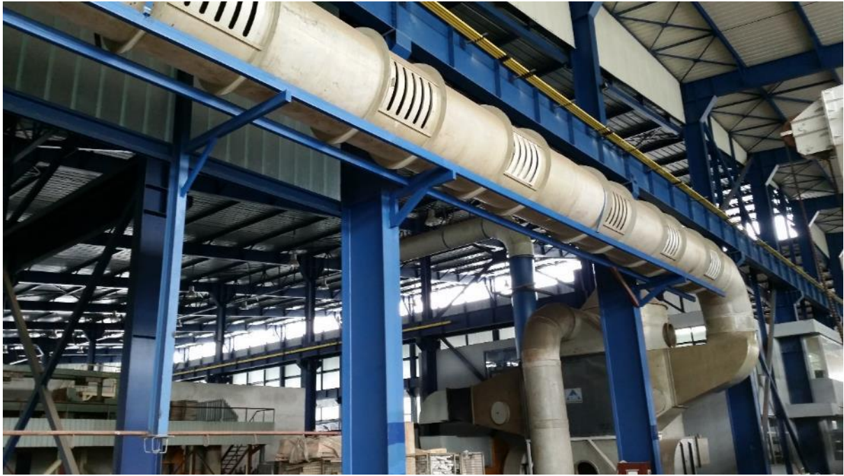
Unit for heating the hall
