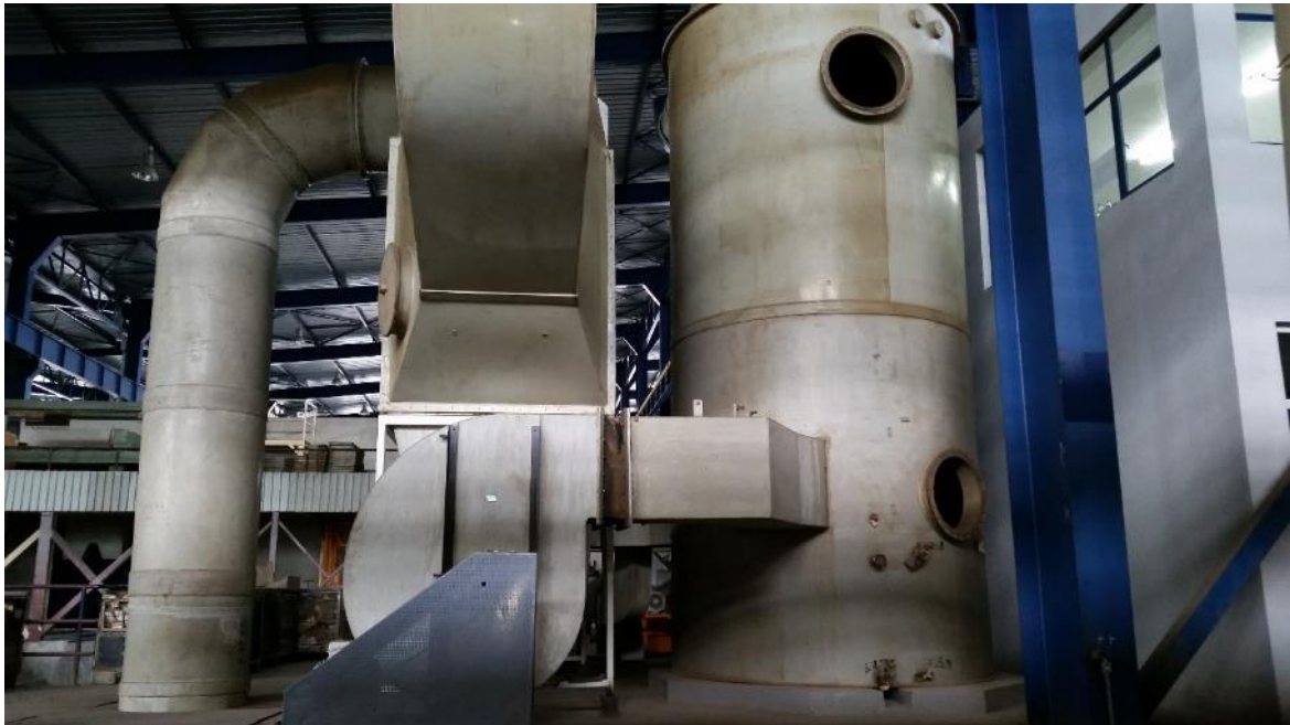
Wet Scrubber & recuperator
