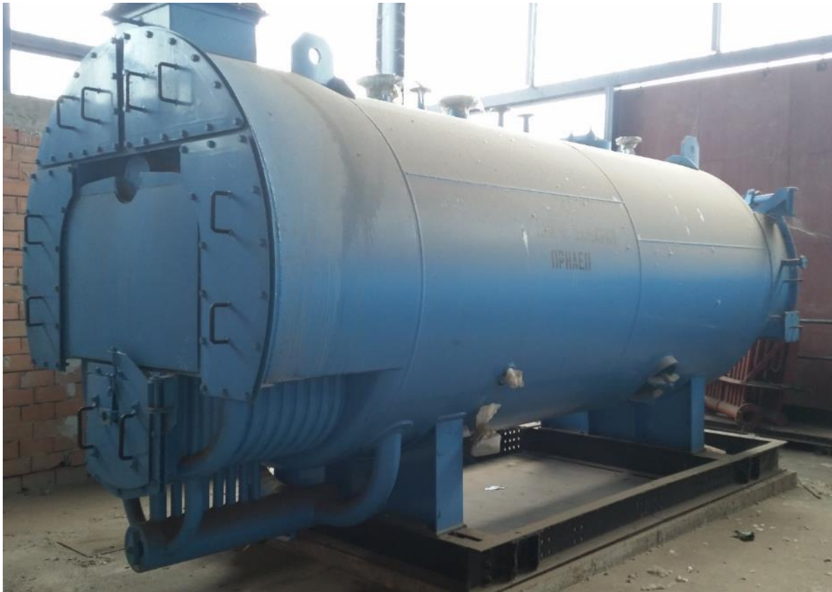
Boiler – Dimce Banjarot
