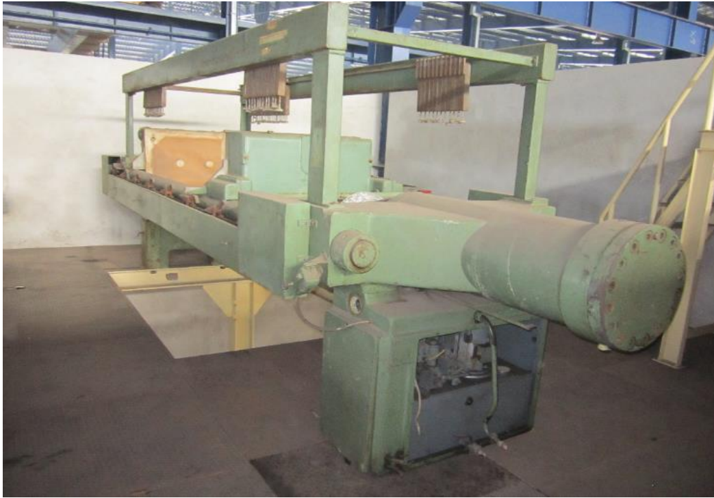
Filter press – Water neutralization plant
